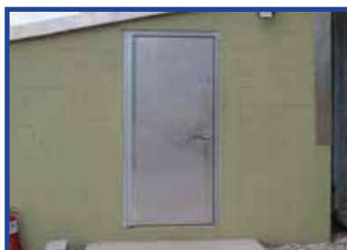
Mechanical Room Flood Door (PD-525)
